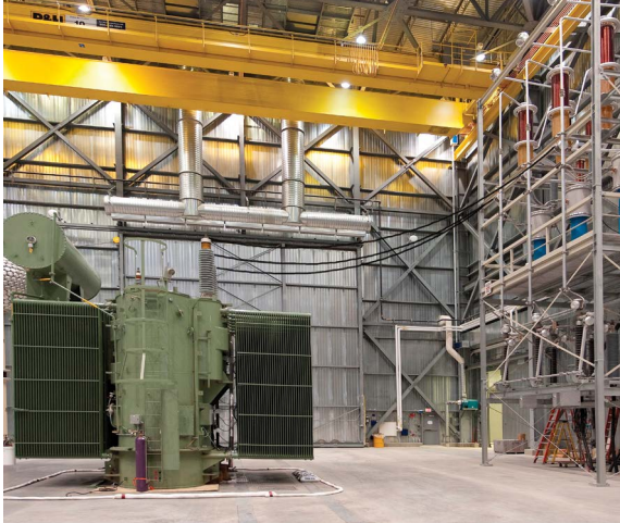
Preparing a 138 kV 125 MVA power transformer for testing. On the right side is the three-phase variable frequency power transformer test system.
