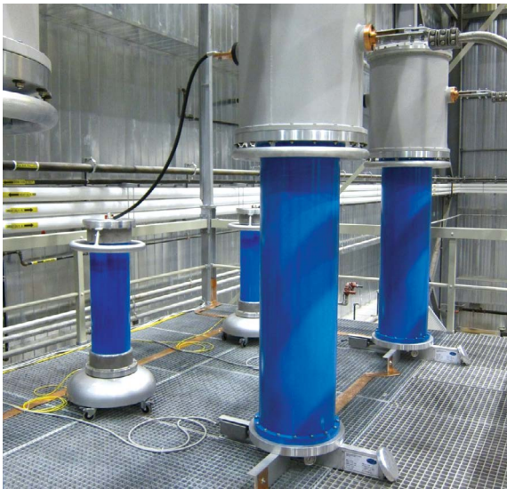
Instrument transformers for loss measuring system.
